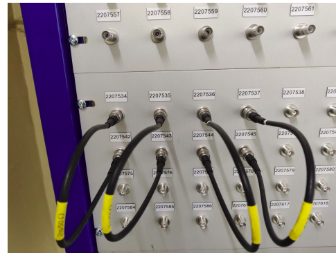
Patch panel NEAR: 2x ~100 m connections
