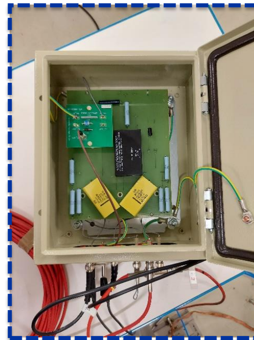
Fig 20. Beam Switch Box finalized.
