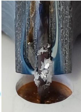
Oxidation at Outlet side
