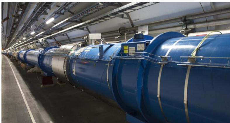
LHC dipoles (8 T) in the tunnel
