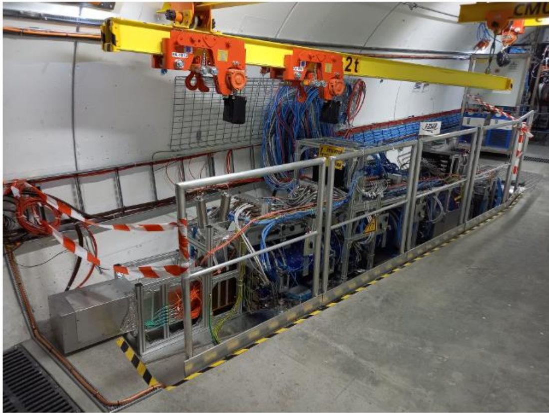
Figure 64: The FASER detector after installation in TI12.
