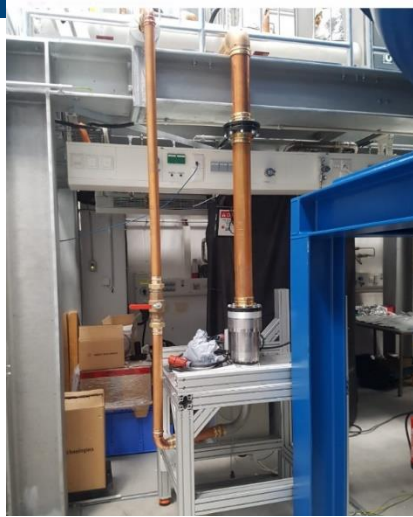
Turbine outside tank
