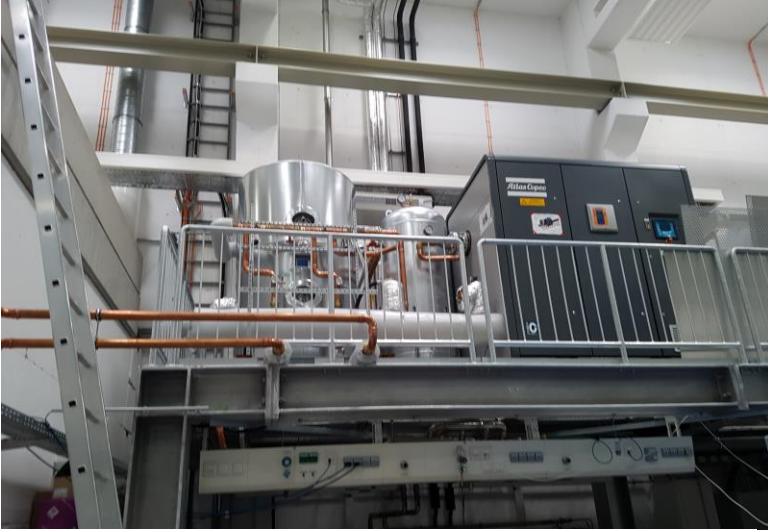
Compressor station for up to three turbines
