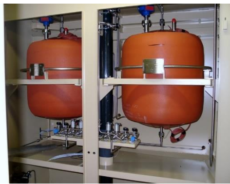
Optical fiber production gas cabinet – PIRELLI cavi (2003)
