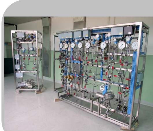
Realization of gas distribution panels for VEGA launch PAD – Korou (French Guyana)
