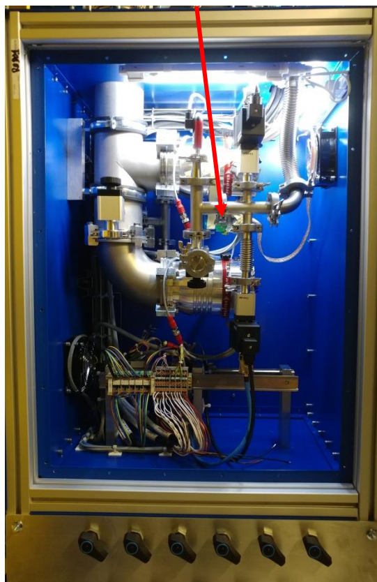
Temporary magnetic sensors
