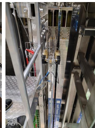
Top gas multiplexer
