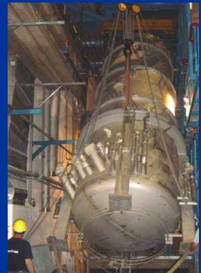
15000 liter nitrogen phase separator
