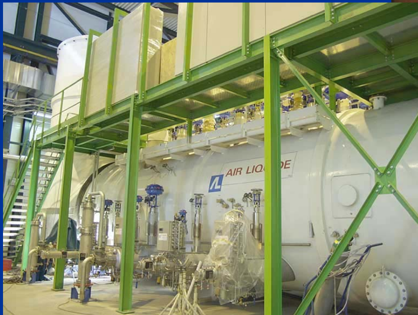
Air Liquide cold box
