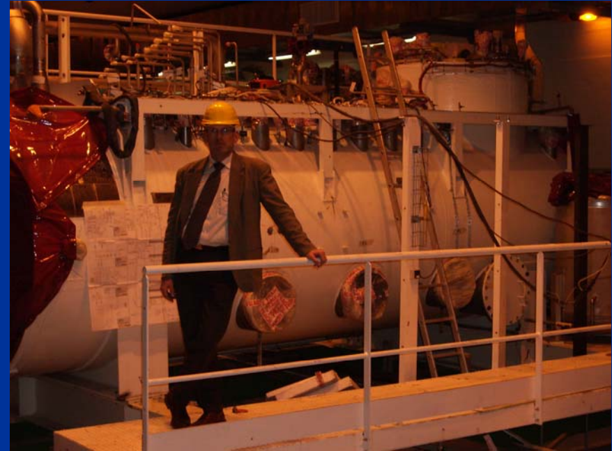
1.5 kW @ 4.5 K Refrigerator cold box installed in underground cavern
