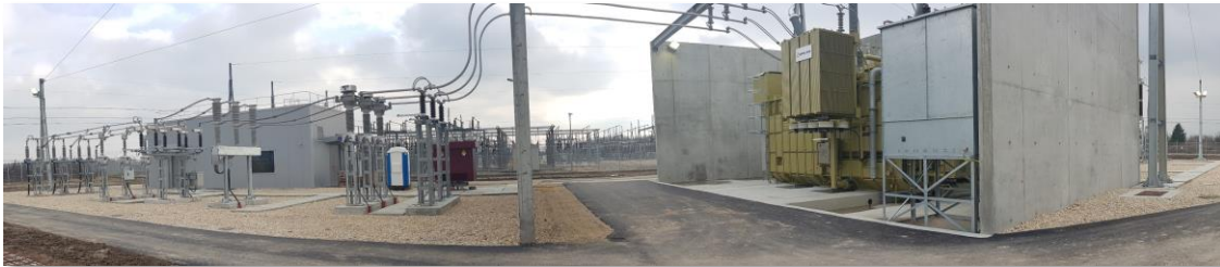
New 400/66kV BE2 sub-station
