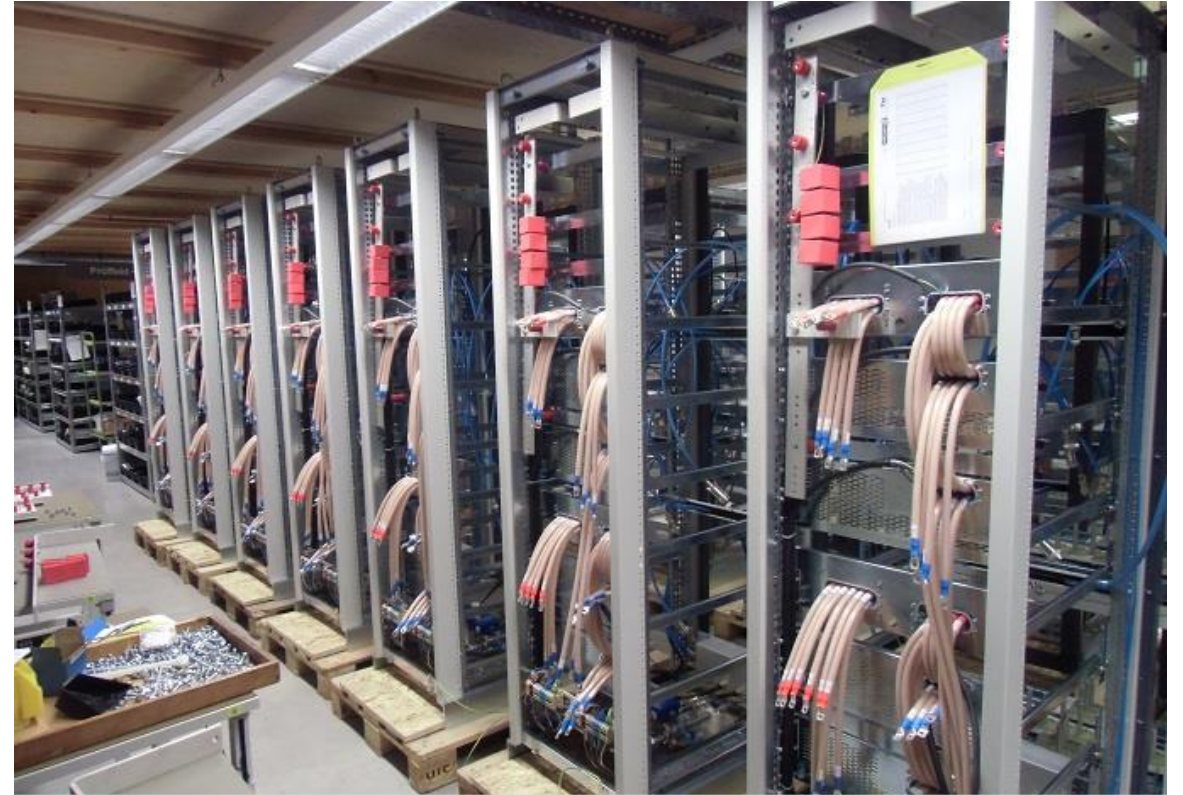
Typical Rack Series Production
