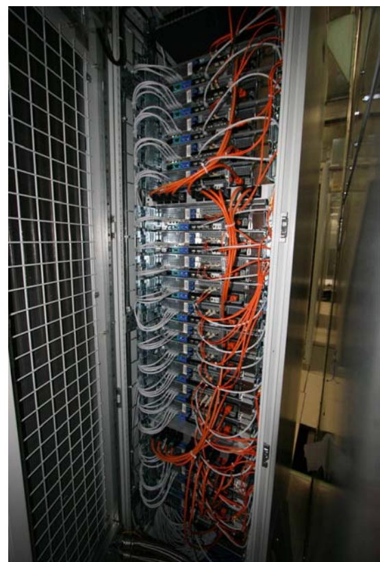
Figure 7: One RUBU rack fully cabled
