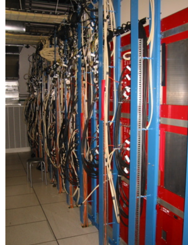
Figure 5: The front of the RCT Racks. Additional, temporary cables seen are for testing.
