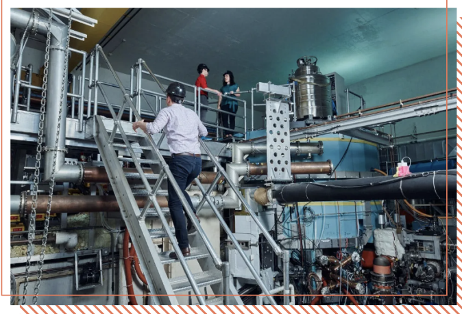
Water cooler talk, except at Commonwealth Fusion Systems it's by the plasma-confining tokamak reactor.
