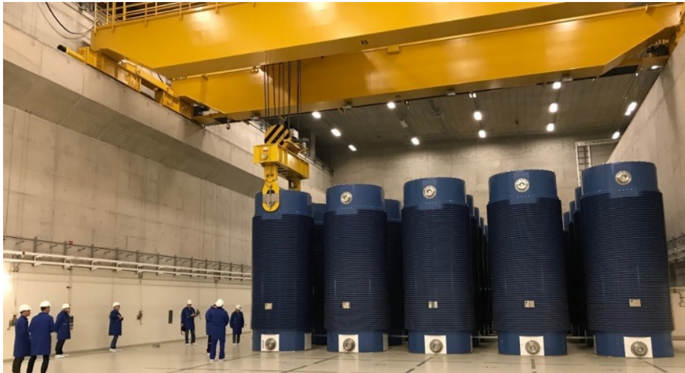
Spent Fuel Storage Casks in an interim storage facility in Germany 4
