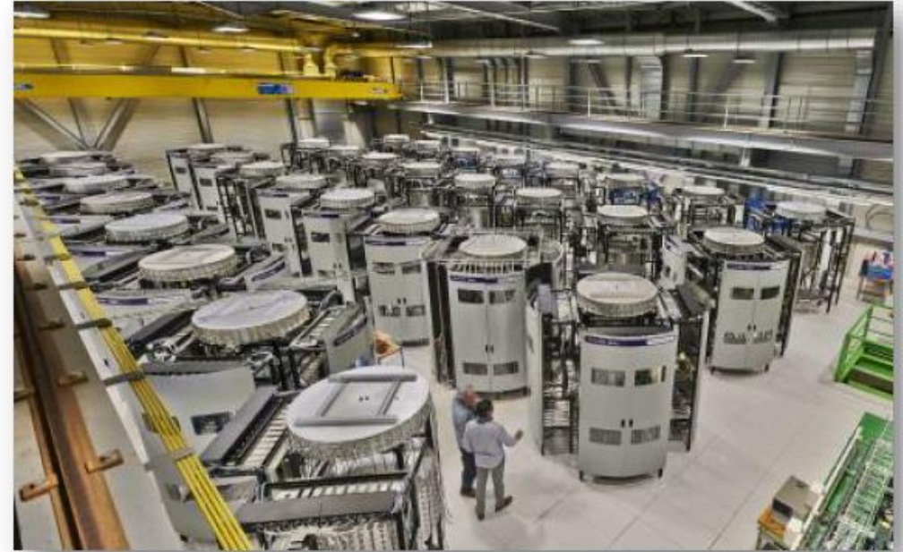
CERN SPS Thales Solid State Power Amplifiers,
