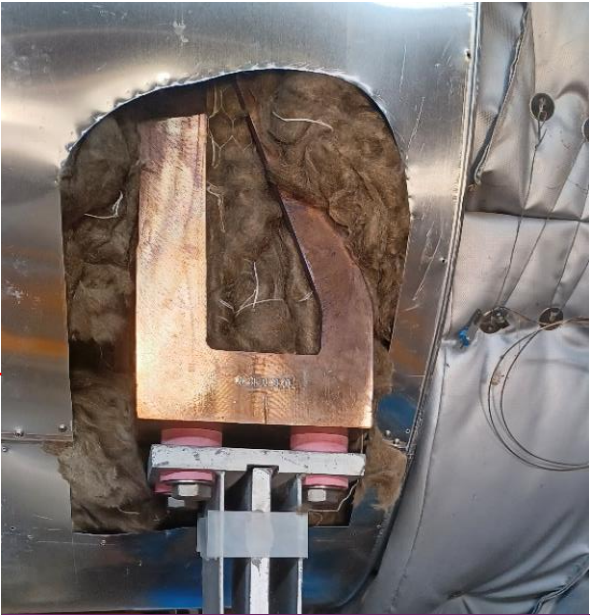
I. Electrical isolation of beampipe stands & covers
