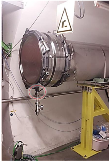
LHC dump windows
