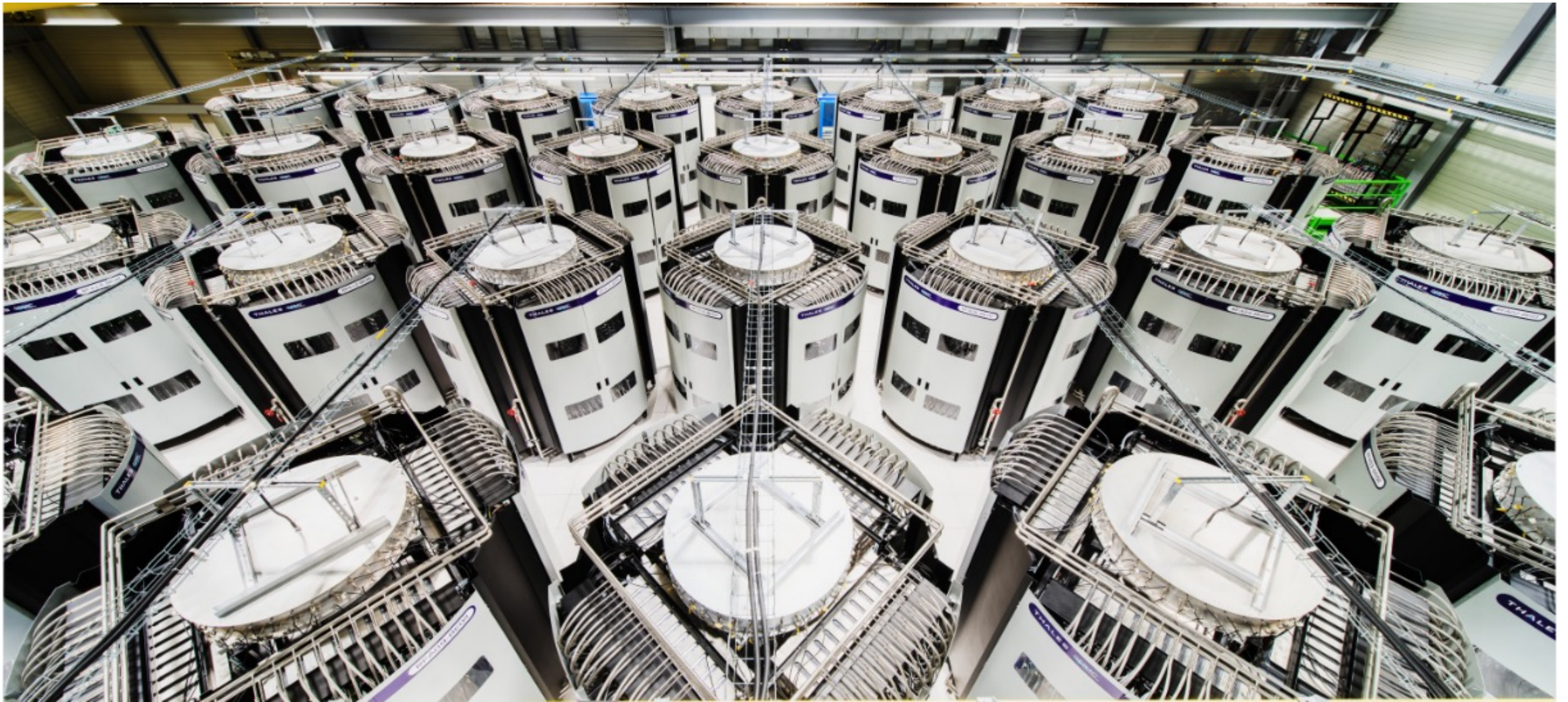
CERN 2 x 16 x 160 kWp @ 200 MHz tower solid state amplifiers (2022)
