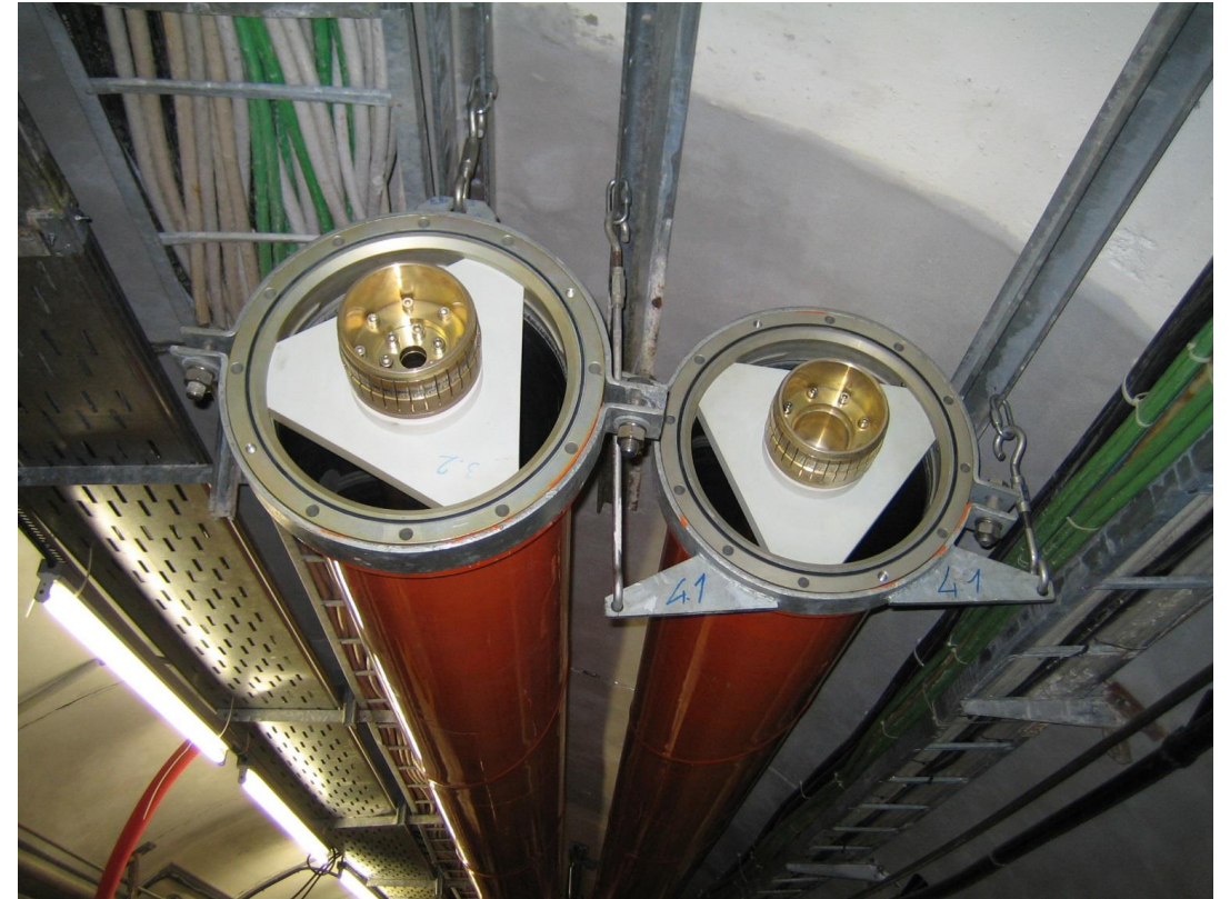
The supporting system is made to allow for movements due to thermal expansion
