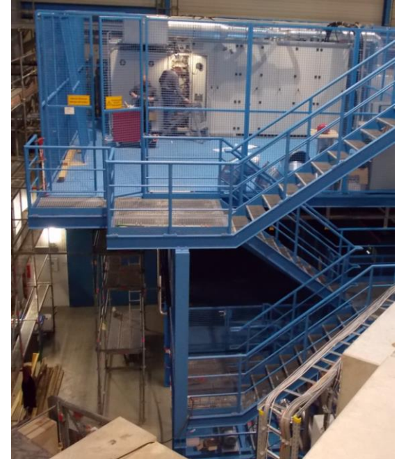
Platform for SIS18 h=2 power supplies (2 nd floor), mains distribution (1 st floor), and oil cooling system (ground floor)
