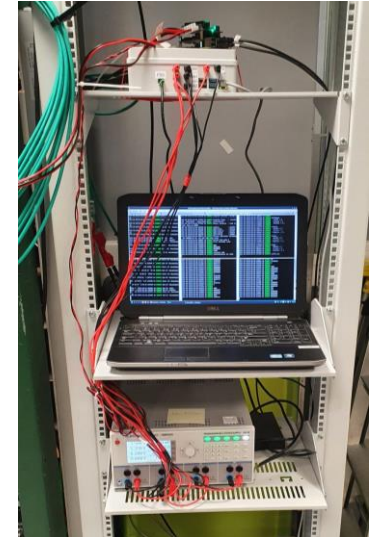
CHARM Control room
