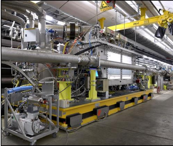
Crab cavity prototype installed in SPS
