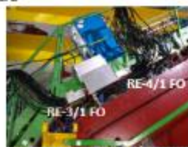
Fiber optics box installed back of VE-3 and VE-4
