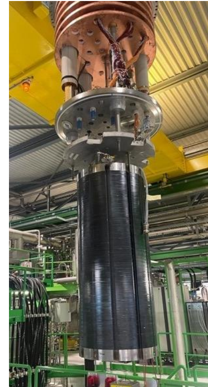
MCBXFB ready to test at SM18 (CERN courtesy)
