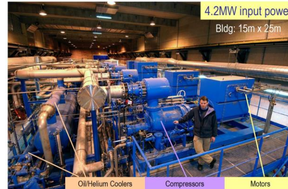
Compressor station of LHC 18 kW@ 4.5 K helium refrigerator
