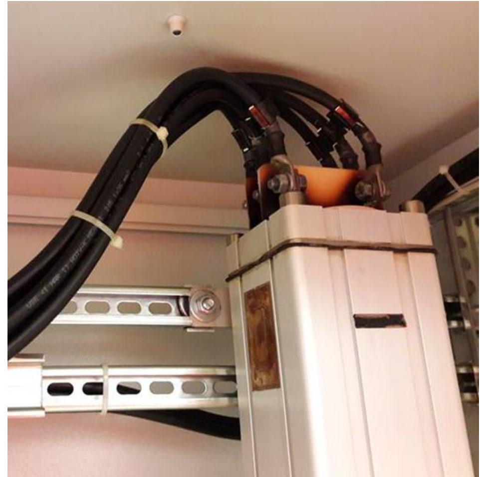
Family D2 PCO sinus filter resistor installation
