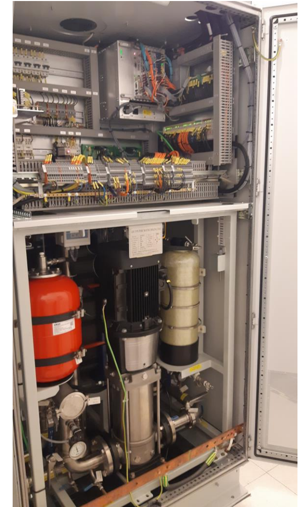
Family E1 PCO output cooling cabinet
