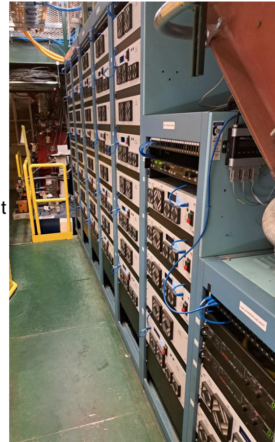
S800 Beamline PS (located in S800 Vault)
