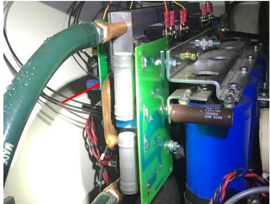
Pin Hole Leak
