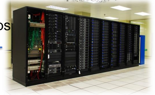
The large Offline Data Center at IHEP
