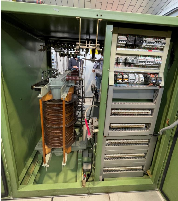
Converter exposed rack with MV transformer on the left
