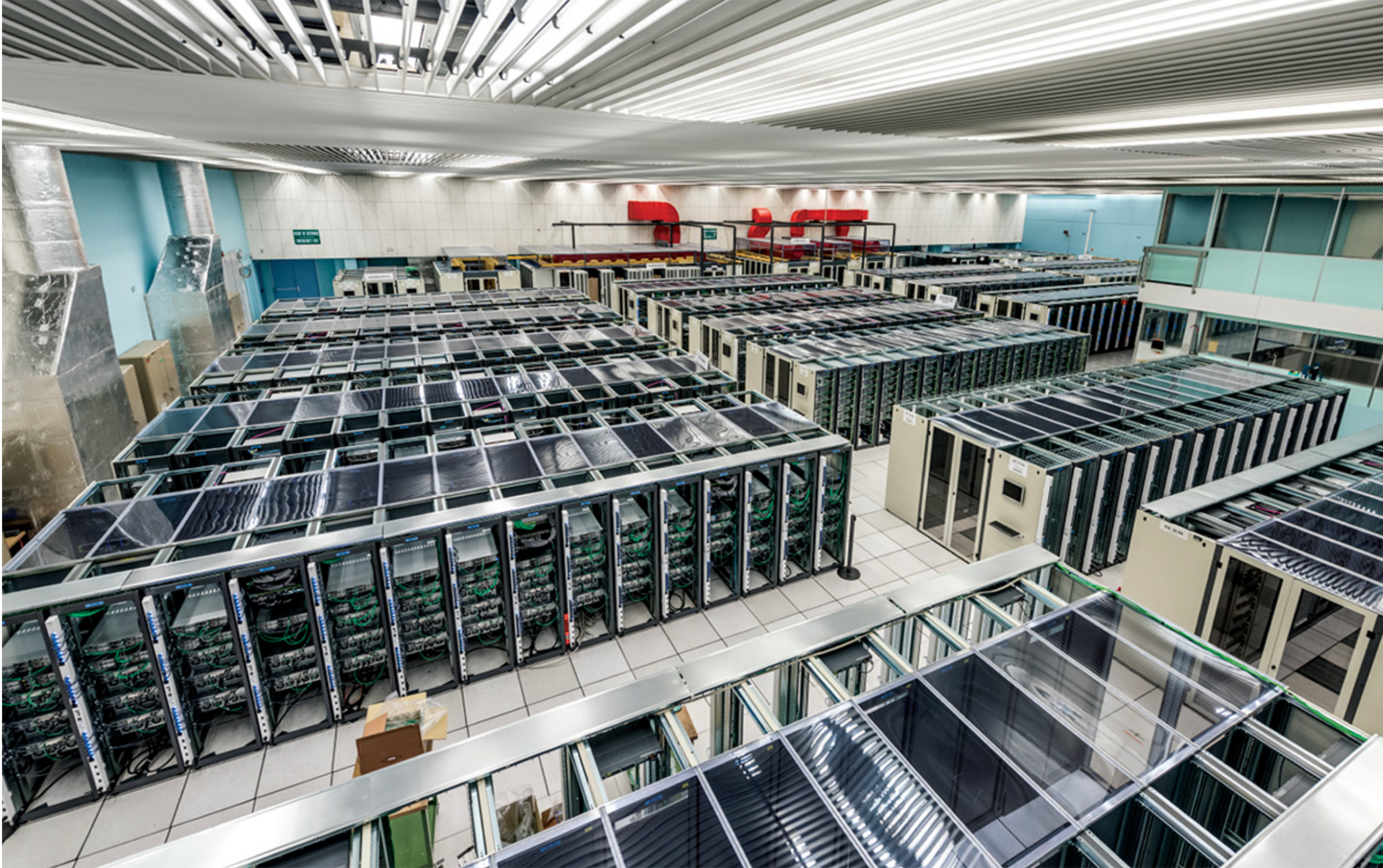
CERN data centre, 2016
