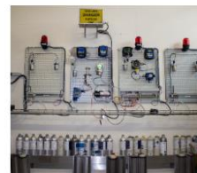
Test platform for detecting gas (including ODH). The bottles at the bottom of the image contain different types of gas used for tests.
