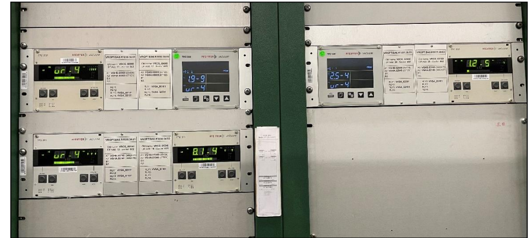
TPG500s installed in BA6
