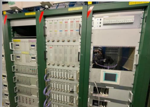
UPS powered racks
