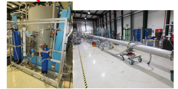
Cleaning facility by circulation
