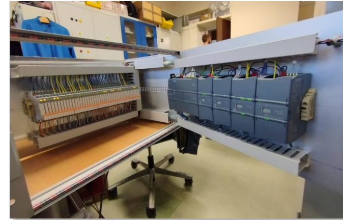
BGC PLC controller
