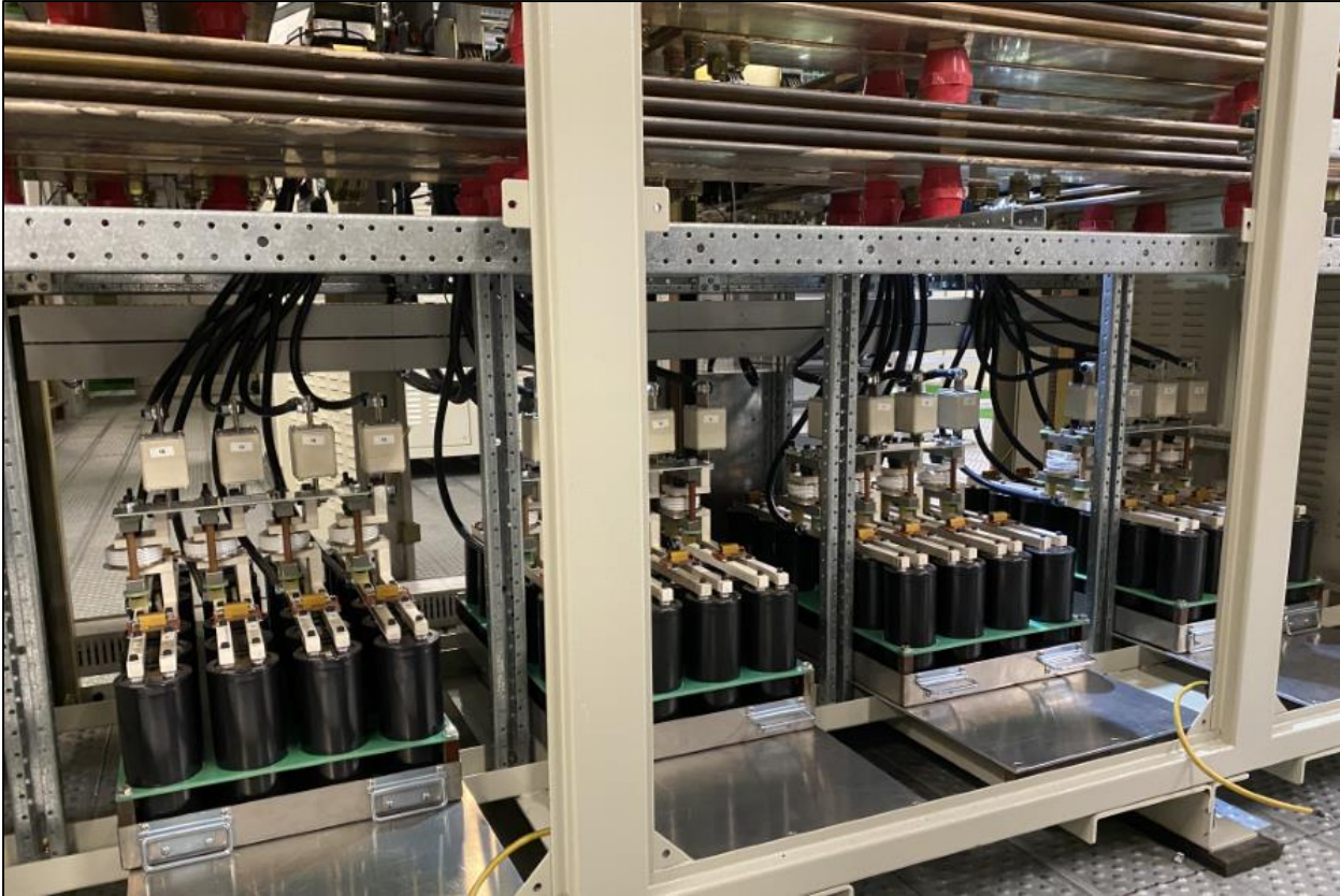
Snubber system for ATLAS Toroid circuit, for arc-suppression during slow-dumps
