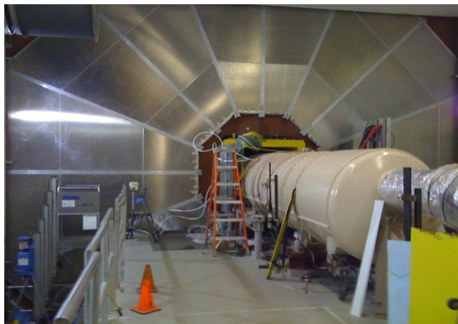
HIM2012 RPC3N - installation (Nov. 11 th , 2009)
