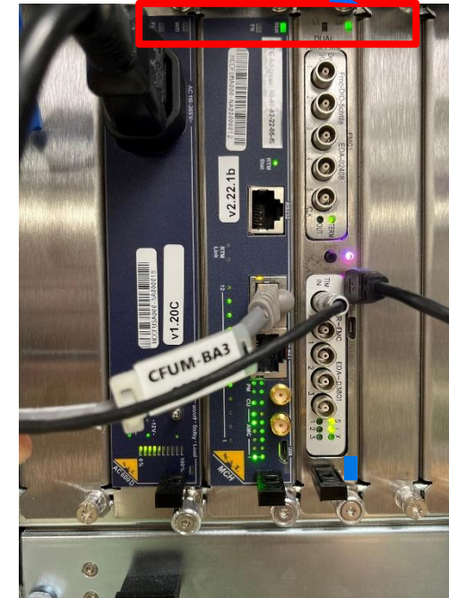
Fig – Power supply, MCH
