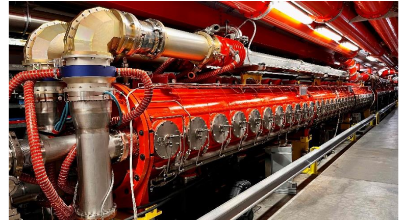
Fig – TWC 200MHz Cavity
