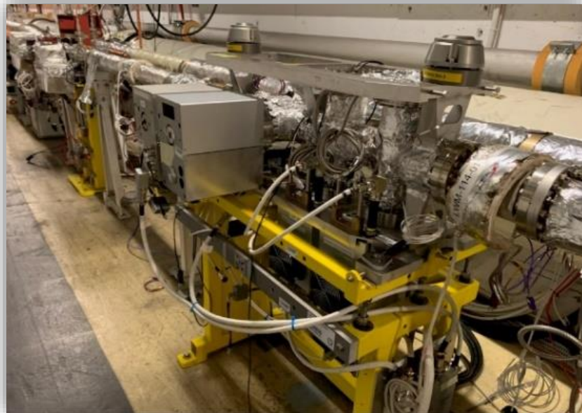
E5R4.B (inner beam pipe)
