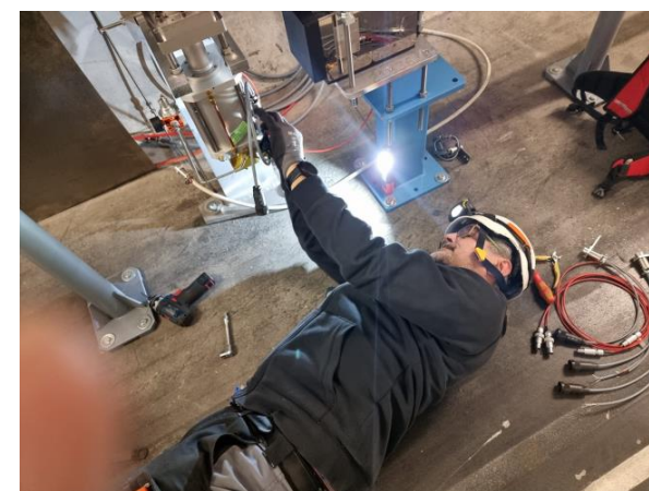
Sector valves consolidation
