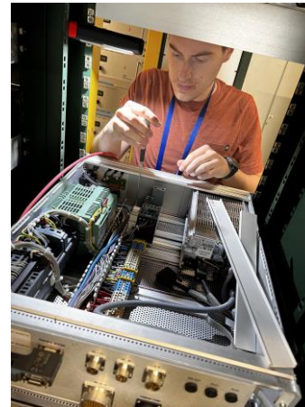
ITL VPG troubleshooting
