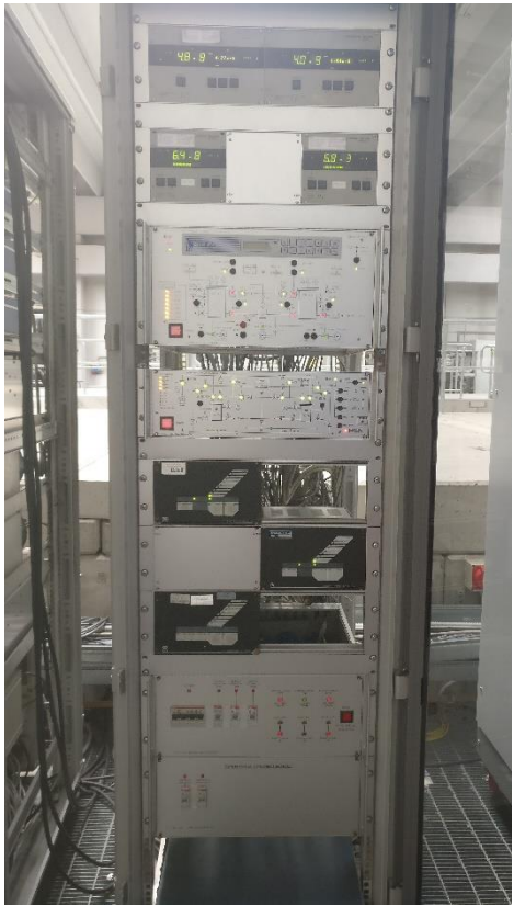
TELEMA Vacuum Control System Racks
