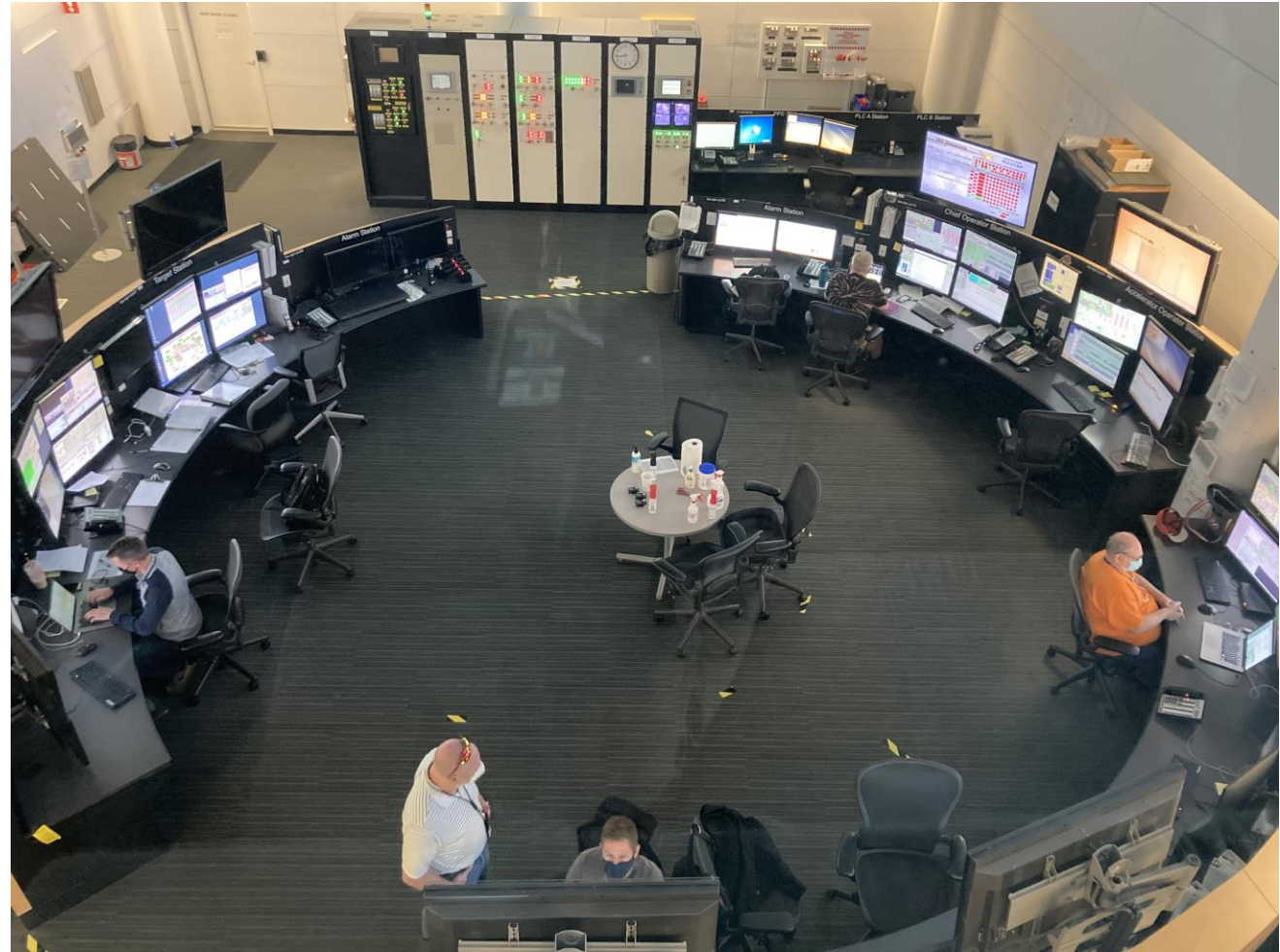
SNS Central Control Room
