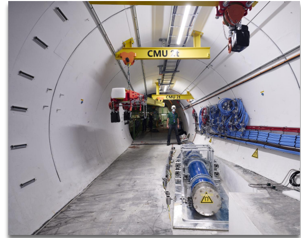
FASER installation in T112 tunnel
