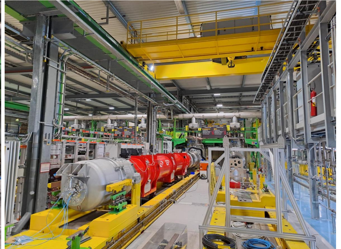
LQXFA01 (Q3 in IT String) placed on bench for cold tests
