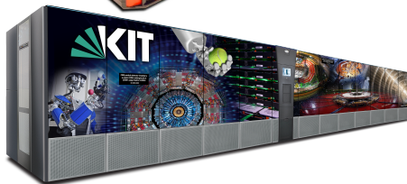
top: tape cartridge & drive, bottom: tape library at KIT (current total capacity: 169 PB)
