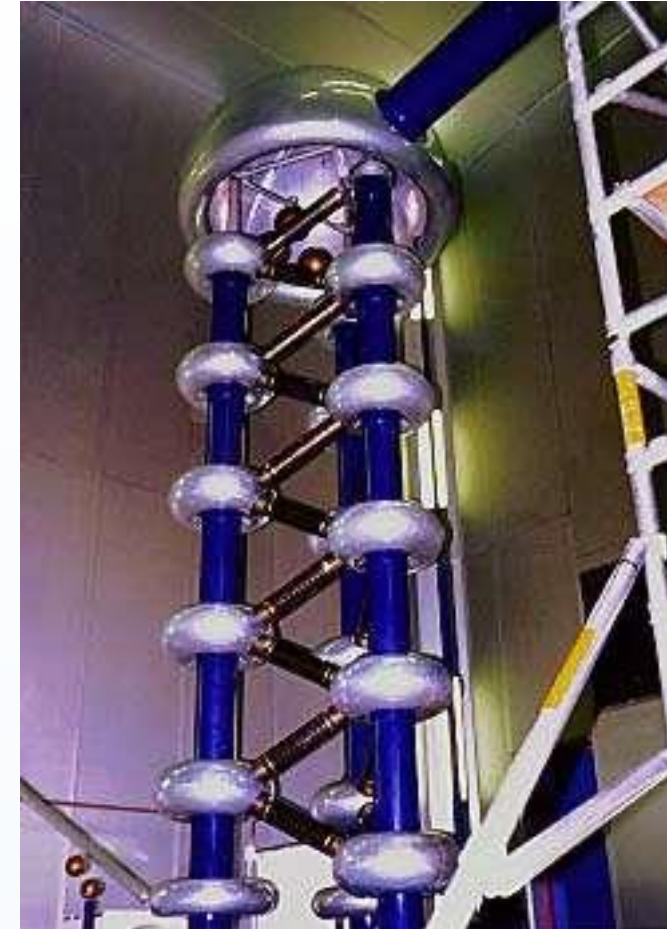
Fermilab cascade generator
