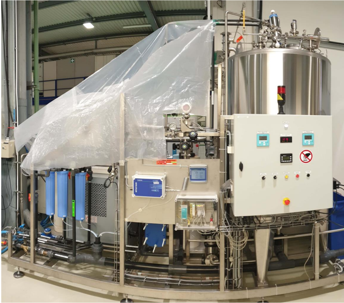
Ultrapure water plant Resistivity (25 °C) > 18 MΩ·cm
