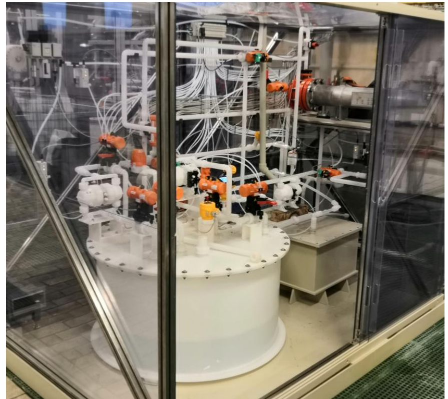
BCP installations at CERN
