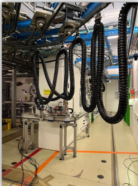
The Montrack conveyor connected to the patch panel with a cable chain.
