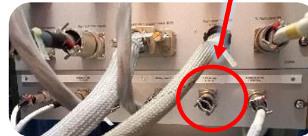
WIC rear patch panel in P1
