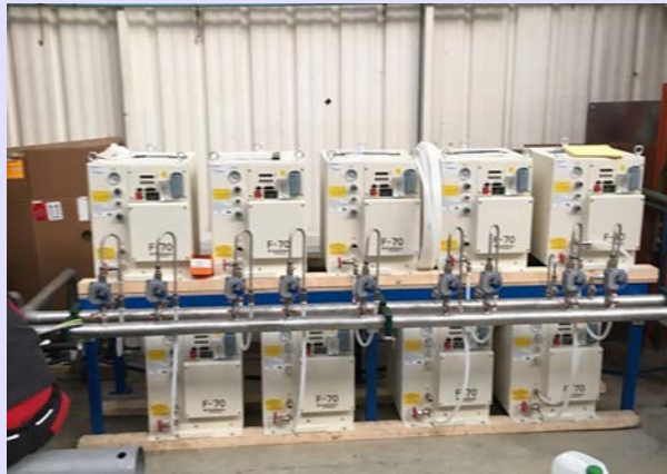
GM cold-heads & compressors
