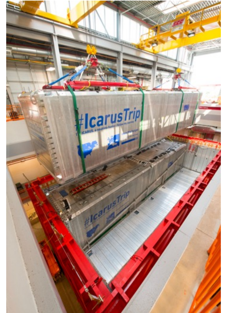
ICARUS installation at FNAL FD
